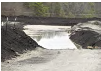
This septic disposal site consists of three or four trenches 250 feet long, 20 feet wide and 8 feet deep in an abandoned industrial waste pit above Spence Branch of Milo. (Citizen photo by Roger Smith)
